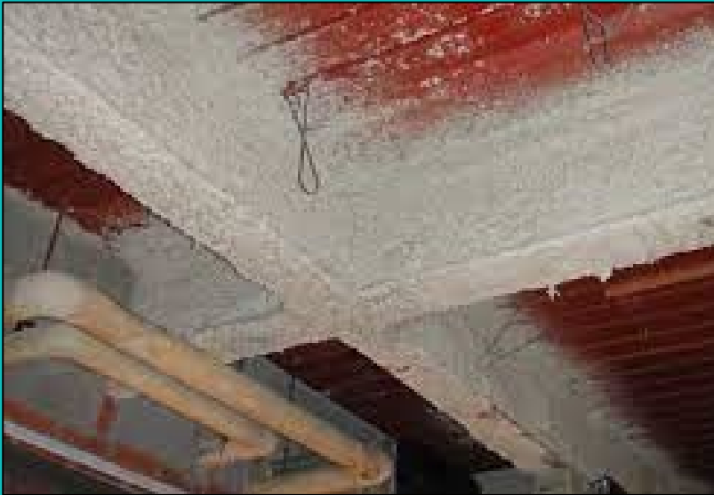
Sprayed insulation / Limpet
