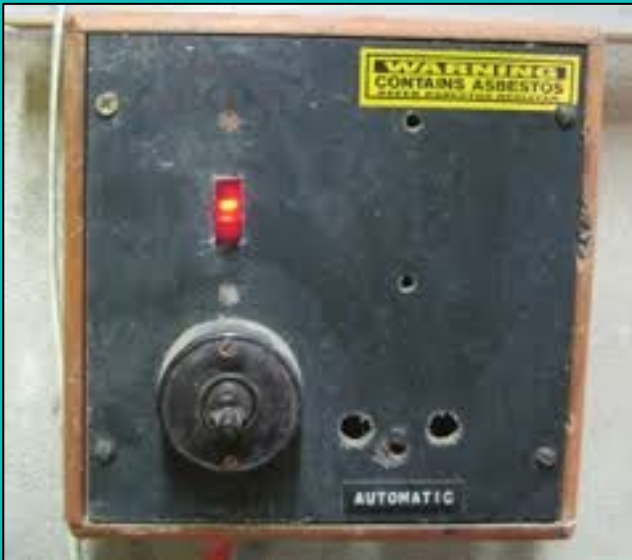
Fuse board backing
